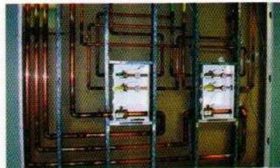
Medical Gas Pipeline
