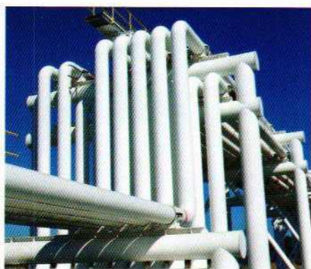
Industrial Gases Pipeline
